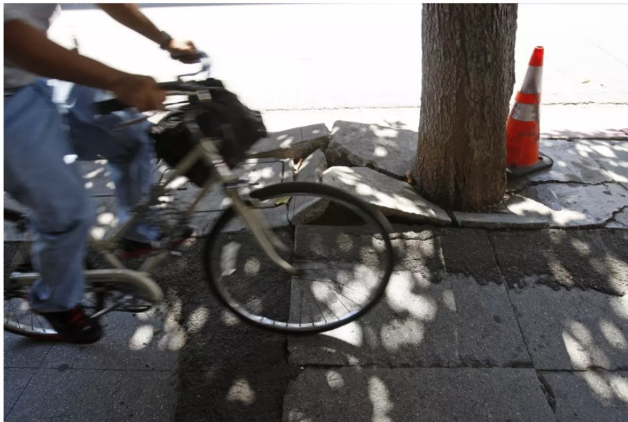
A buckled sidewalk at 4th and Main streets in downtown L.A. (Gary Friedman / Los Angeles Times)
